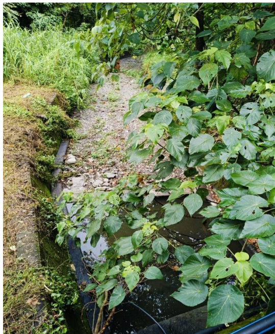
路面龜裂下陷潛在風險
